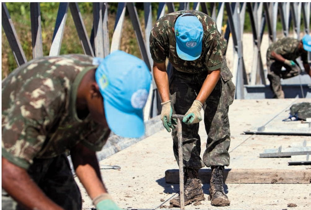
Members of the Brazilian engineering battalion of MINUSTAH assemble a bridge to improve access to Boucan Carré, a small village 60 kilometers north of Port-au-Prince, in October 2009. UN Photo/Marco Dormino.
