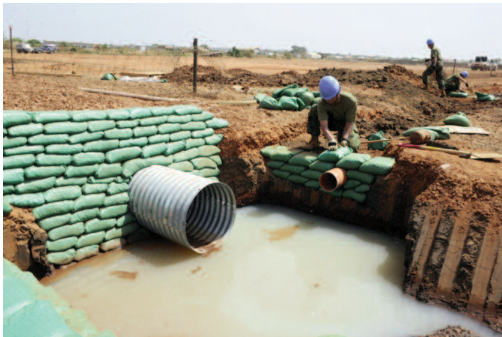
A team of Japanese engineers helps the government of South Sudan with road construction activities in Juba in February 2012. UN Photo/Isaac Billy.
