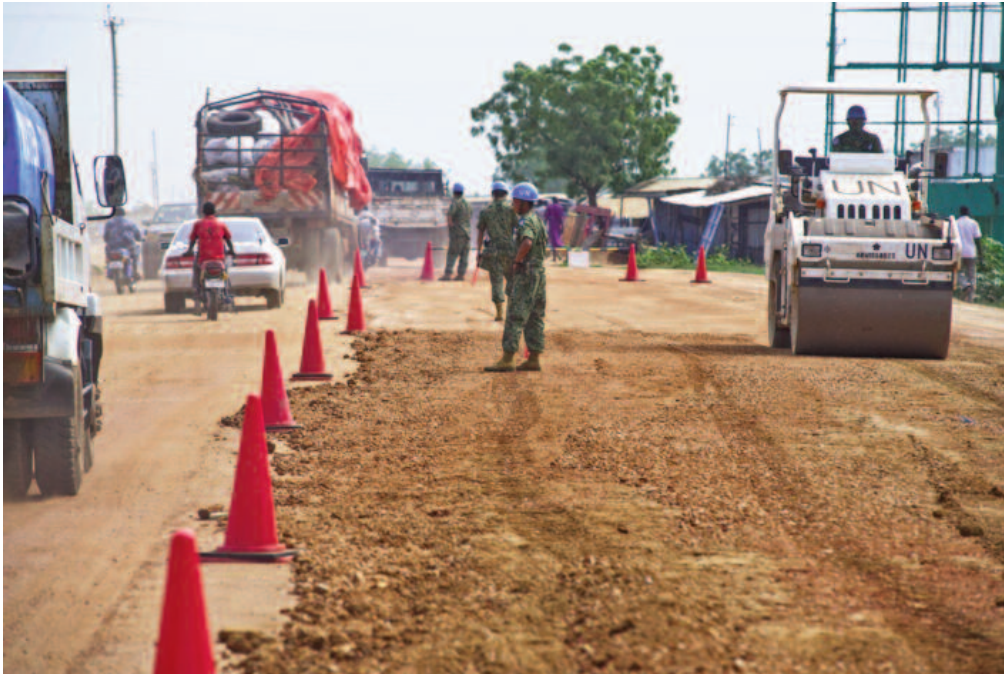
Japanese engineering peacekeepers serving with UNMISS upgrade Yei Road in Juba in August 2012. UN Photo/Staton Winter.
