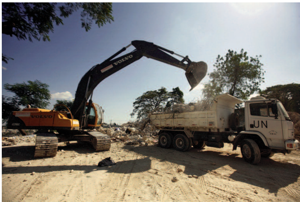
Brazilian military engineers with MINUSTAH use dump trucks to dispose of the debris from their former base in Bel Air, Port-au-Prince, in February 2010. The base collapsed in the January 2010 earthquake, killing seventeen Brazilian peacekeepers. UN Photo/Sophia Paris.
