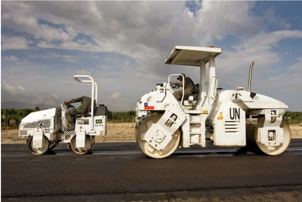
Members of the Chilean and Brazilian contingents of the United Nations Stabilization Mission in Haiti (MINUSTAH) construct a new road to the general dump in Port-au-Prince on September 8, 2009. UN Photo/Logan Abassi.
